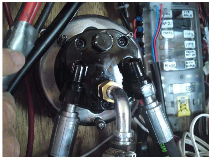
Figure 11 Steering pump, seen from opening in saloon. The middle hose is for overflow from the auto pilot pump.
