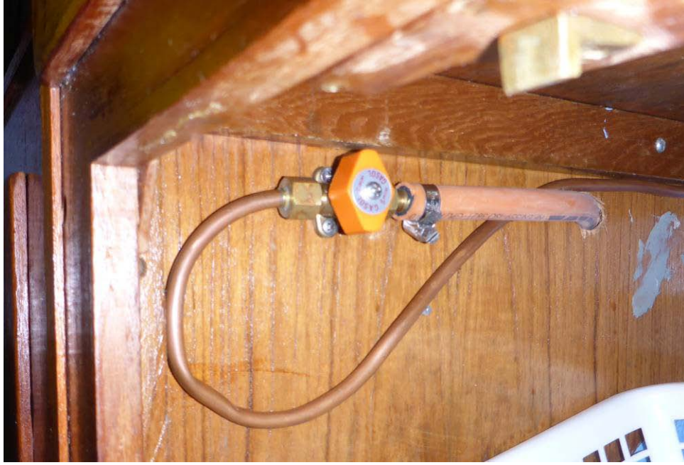
Figure 10 Gas switch just before the stove. The rubber tube goes to the stove. The figure shows the switch off position.
