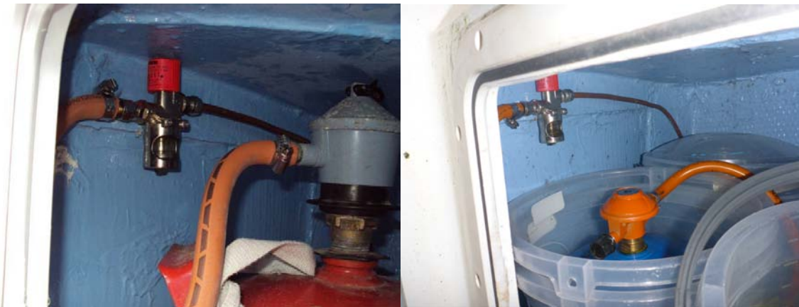
Figure 9 Gas room. In upper left hand corner is seen the leak detector. To the left is a 5kg bottle and to the right a 2kg bottle.
