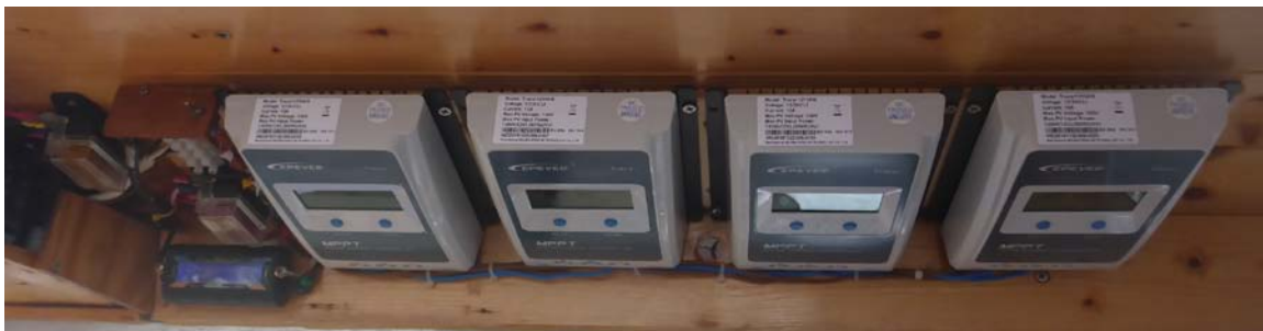
Figure 32 Solar panels regulators. To the left is seen the amp-meter measuring the total charge current from all solar panels and the fuses protecting the panels. The switch is used to turn of the amp-meter. The next figure shows the interconnection.
