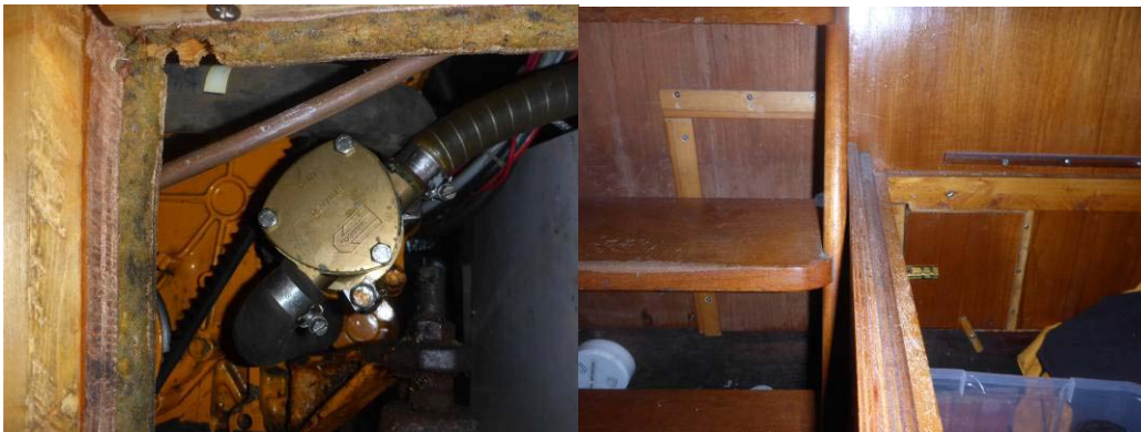
Figure 23 Water pump. To the left is shown the pump and to the right the location of the trap door under the bunk in the saloon.
