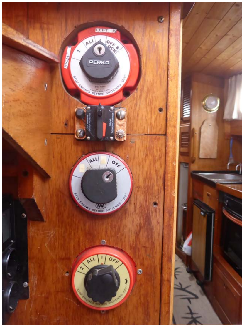
Figure 2 Switches for batteries. Battery 1-2 on top switch, 3-4 on middle switch and 5 on bottom switch. Between the two top switches is seen the main 200A automatic fuse which work on all the batteries.
