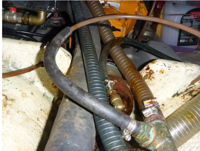
Figure 21 The location of the hose (brown fitted into a black one) to the stern tube for pumping water to the cutlass bearing. The photo is taken from the storage room under the cockpit.
