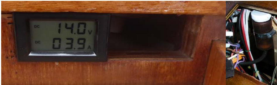
Figure 34 Left: Voltage and current monitoring. Right Below the motor instrument panel there is a brown bottle for topping up hydraulic oil. See also Figure 13.
