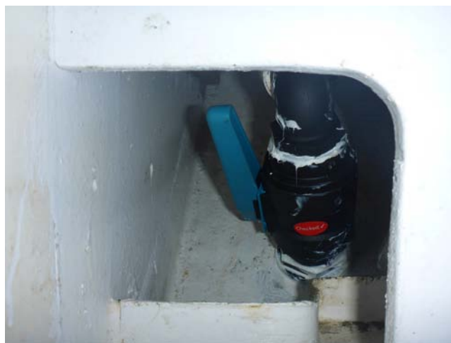
Figure 25 Valve from toilet to the sea. It is shown in the open position. To close, turn 90 degrees.
