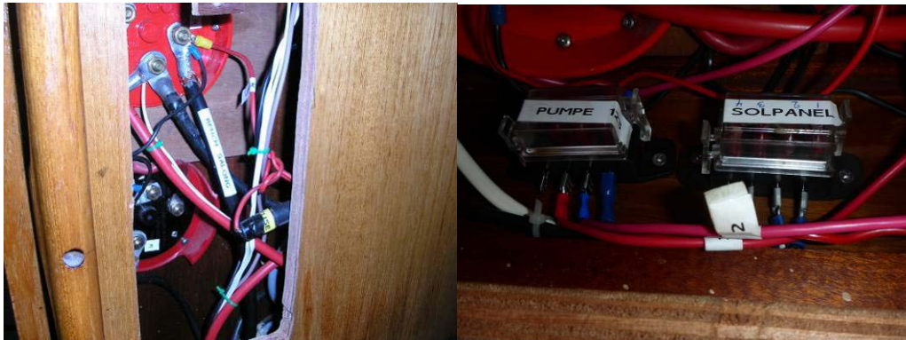
Figure 36 Left: The back of the two main battery switches. Right: Fuse holder for the automatic bilge pumps and fuses for the solar panels (between regulator and battery).
