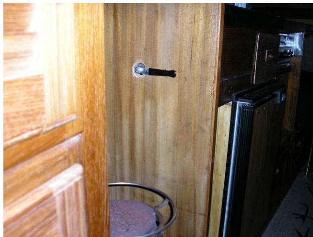
Figure 7 Location of valve for hot and cold water. The handle is in the warm position.
