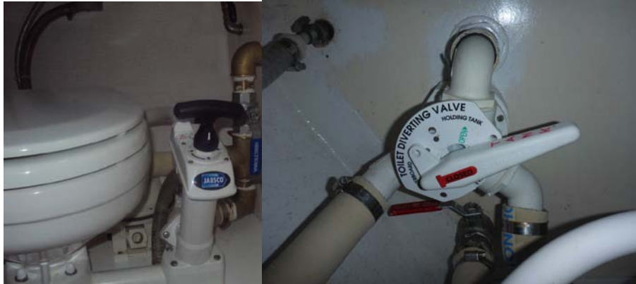
Figure 24 Left: Toilet and pump. Right: Two way valve for pumping out in either tank or sea. The sea water inlet is below the toilet.
