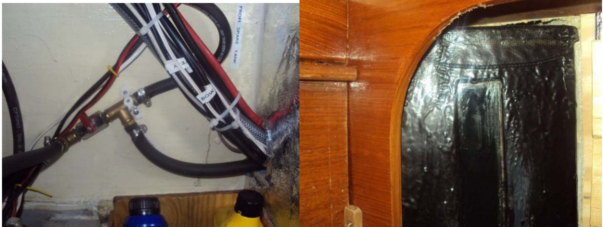
Figure 17 Left: Valve for diverting oil from the spare tank to the motor. The valve is shown in closed position (normal operation). Right: Spare diesel tank in cockpit. Notice the glass window showing the diesel level, normally it should be almost full.
