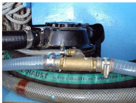
Figure 55 Steering room. The bottom hose is for the electric bilge pump, the green hose is the exhaust and the transparent hose is the output of the cooling water. Note the small hose venting the cooling water hose. All hoses are here above the water level to make a “swan neck” to prevent water to siphon back in.
