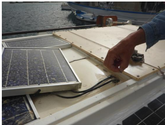
It's here the water is coming, under the solar panel
