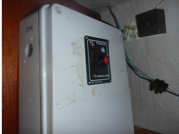
Automatic fuse for the stern winch, in the rear cabin cupboard.
