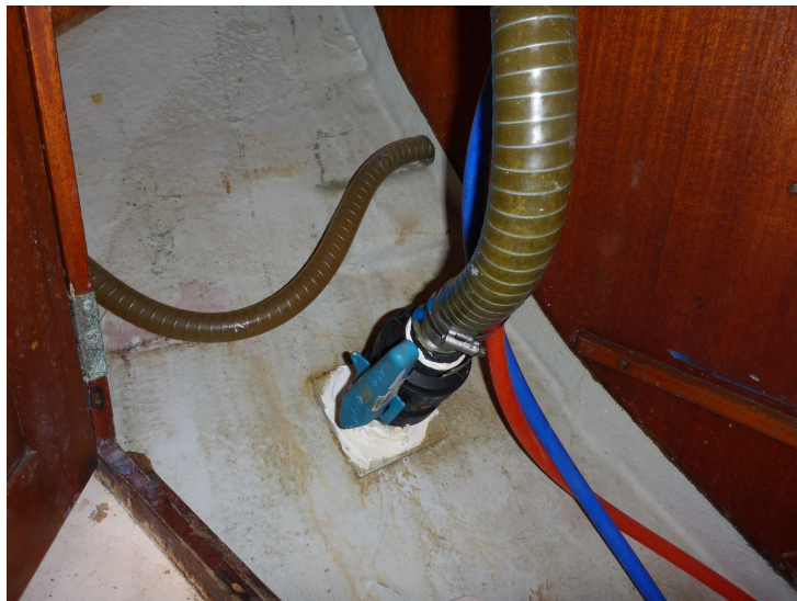
From toilet sink, under the sink
