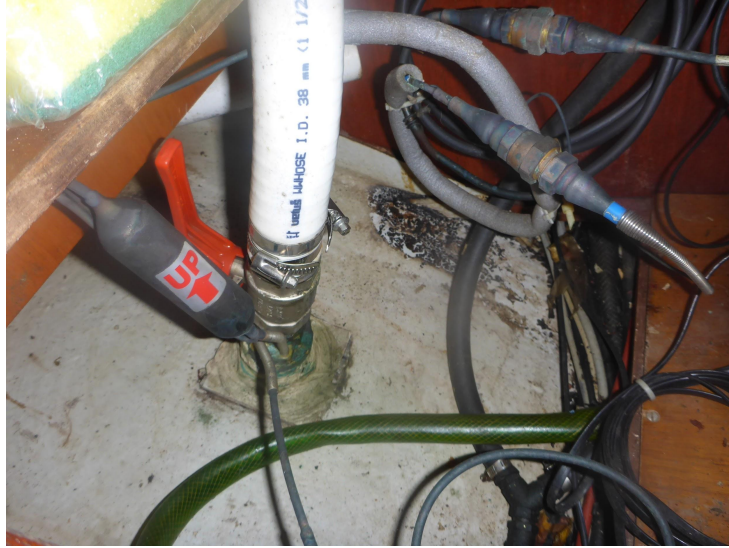
Drain from the kitchen sink, below the cupboard. This is a special hull fitting used for cooling the fridge. It was not changed to composite.
