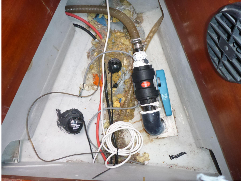
Water to toilet, under floor of front cabin. Also seen is the depth sensor (left) and the speed sensor (front). The loose plastic tube has a plug to put into the speed sensor hole when the speed sensor is taken out for cleaning. The cables are for the bow thruster.
