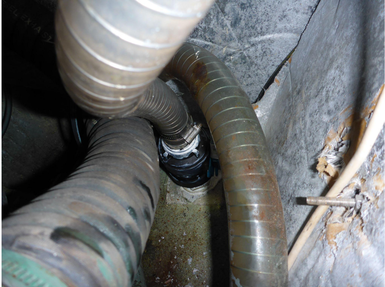
For cooling water, in the motor room.
