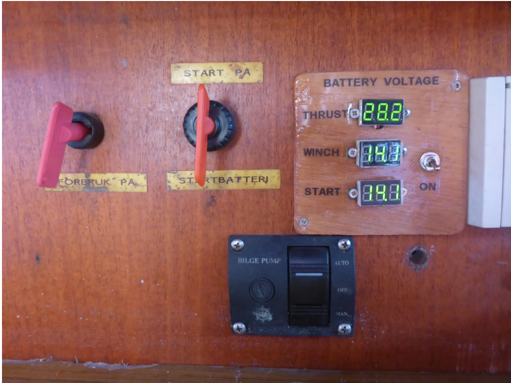
The three voltmeters for monitoring thrust, winch and start batteries.
