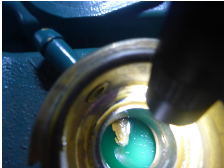
Cooling liquid near the minimum mark, the yellow metal pin sticking out.
