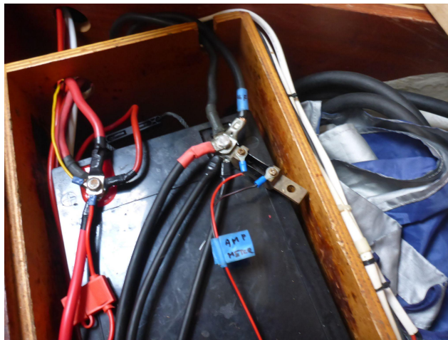
Service battery, the shunt for the ampmeter is seen.
