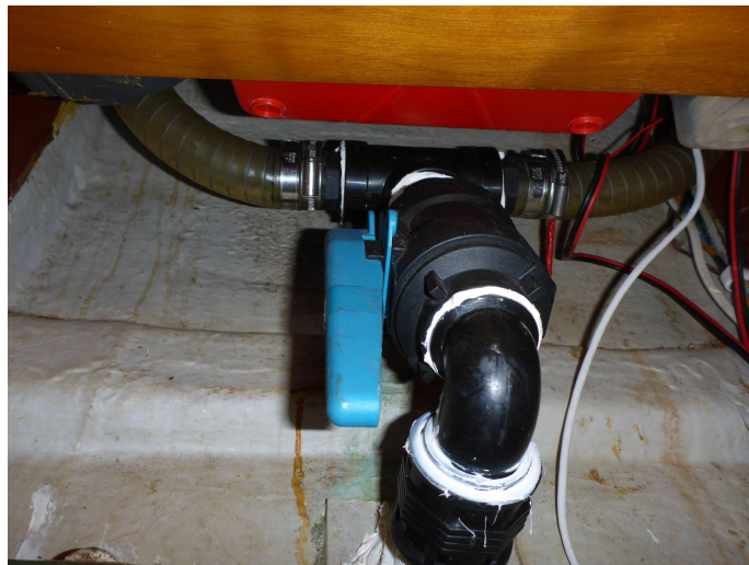
Drain from deck, left side, in cupboard below instrument panel.
